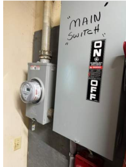
Figure 14-Service Disconnect and Meter
