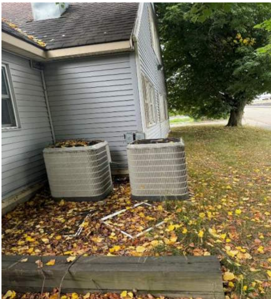
Figure 1 Air Conditioning Condensers
