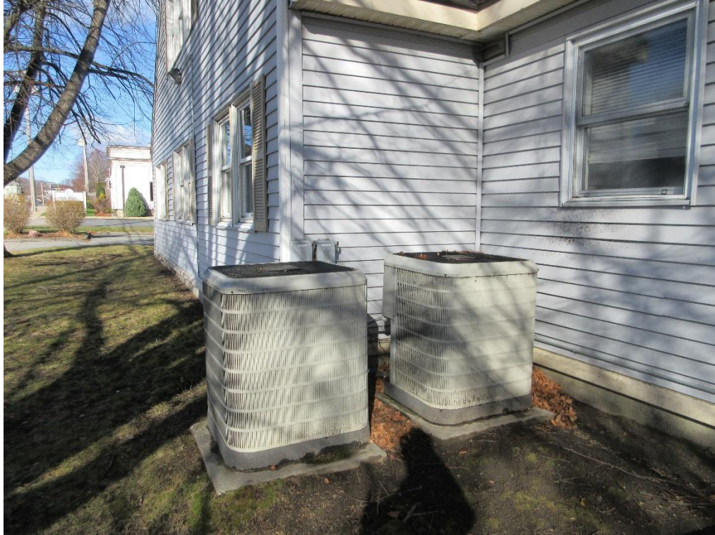
Air Conditioner Condensers
