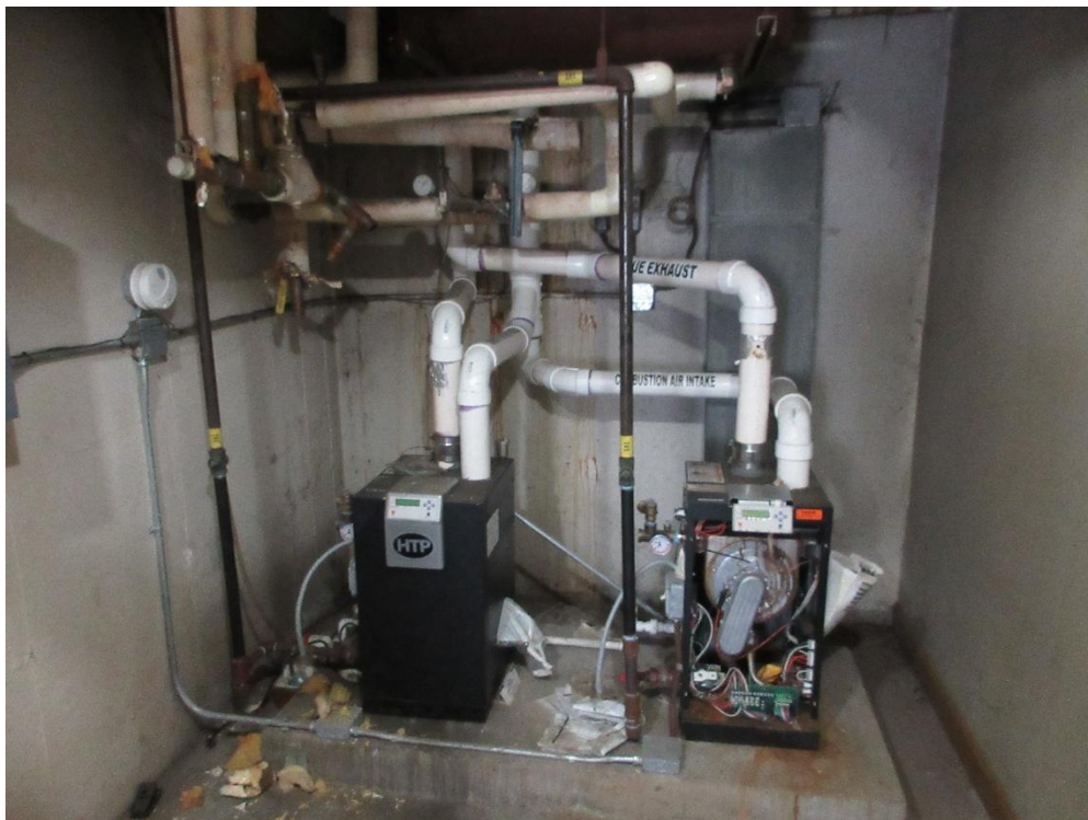
View of Furnace
