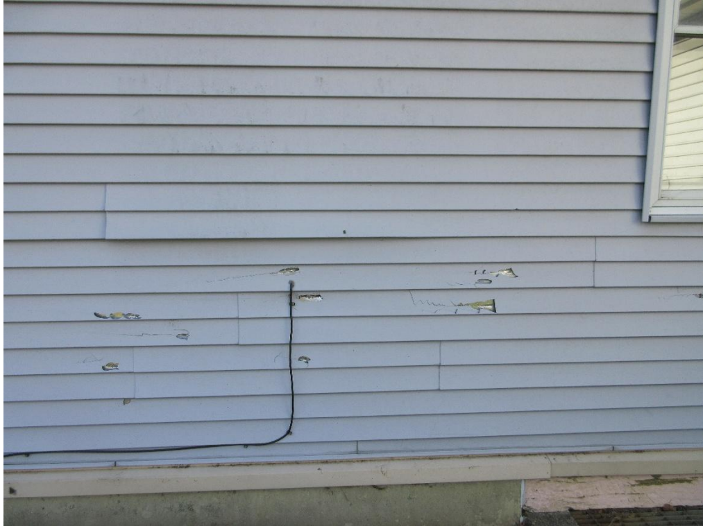
Sample View of Damaged Siding
