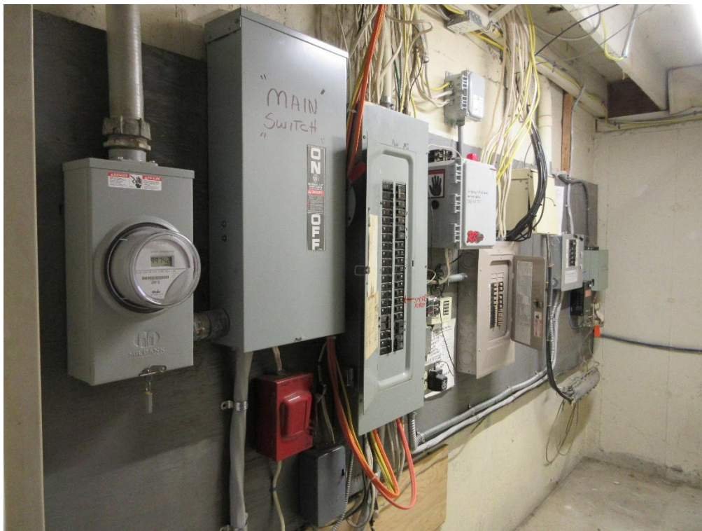
Electrical and Computer Wiring
