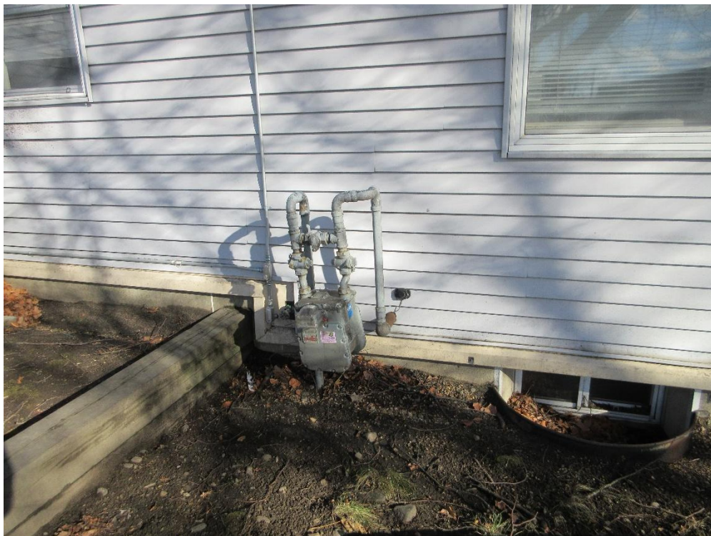
View of Gas Connection
