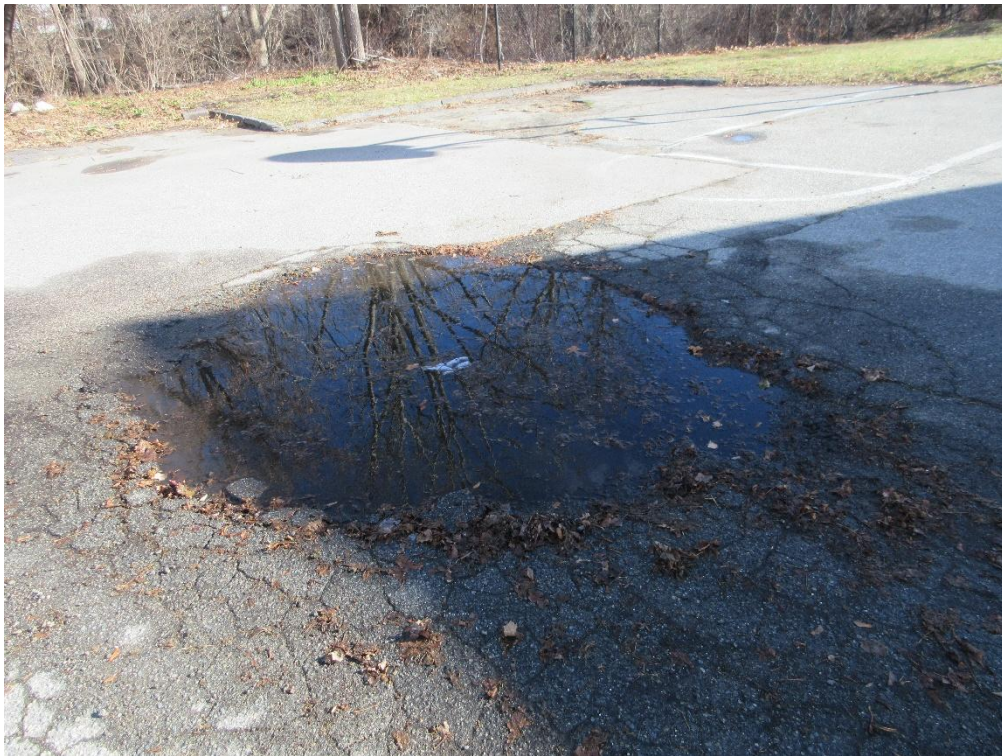
Sample Damaged Parking Area
