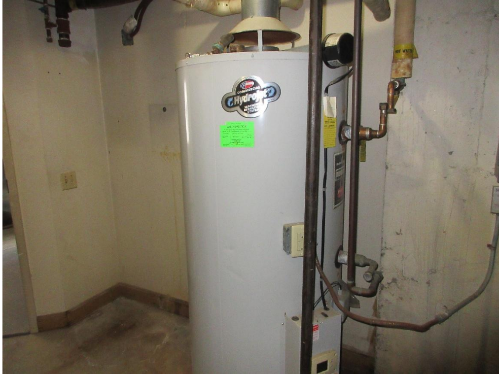
Hot Water Heater
