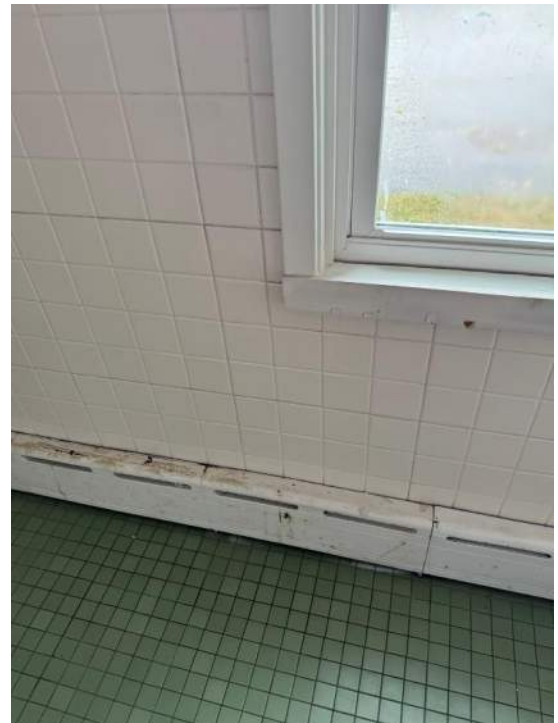
Figure 5- Radiation in Toilet Room
