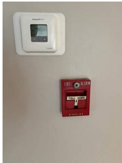
Figure 18-Typical Fire Alarm Device
