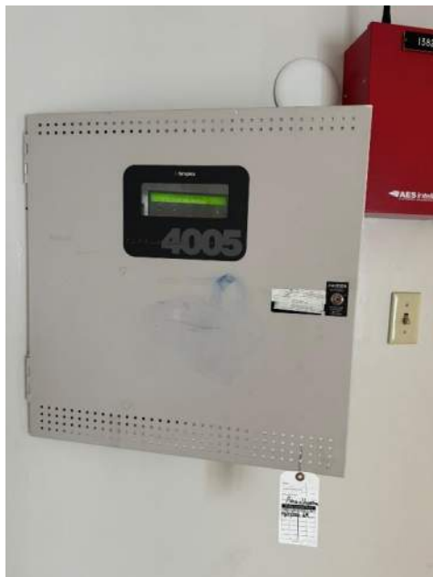
Figure 17-Main Fire Alarm Panel
